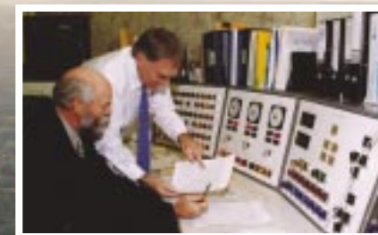
The Leigh Barrier control room
